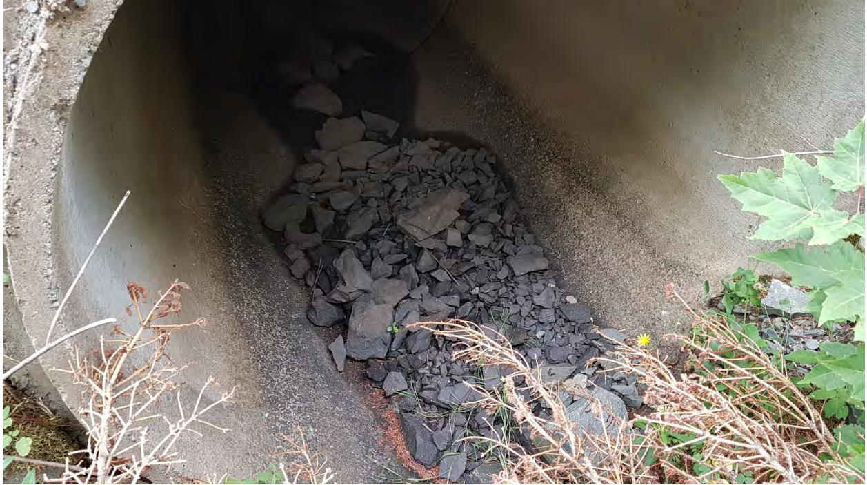
Photo 5. Area 4D – There was no flow in Culvert 1, despite recent rain.
