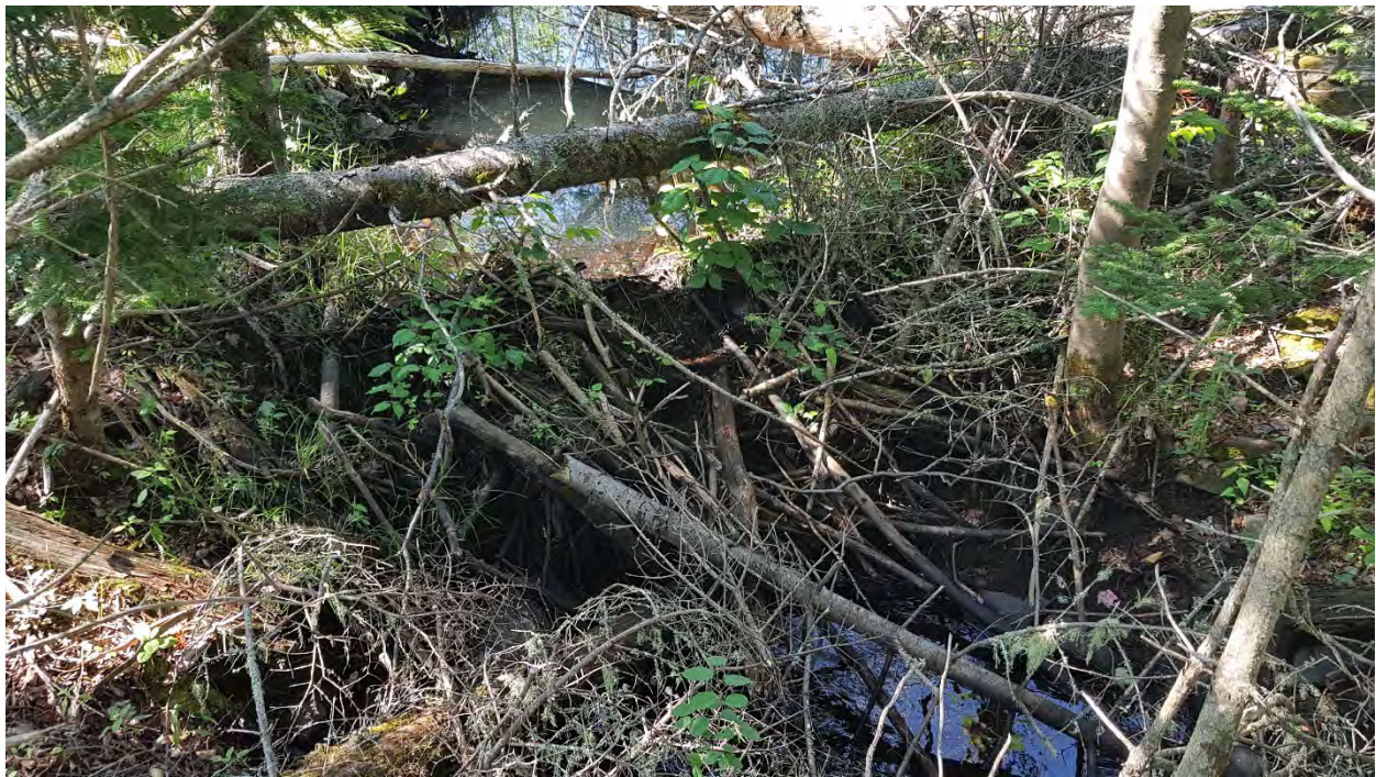
Photo 30. Area 1G – A small beaver dam currently blocks effective drainage in the trench but there is still a significant flow downstream.
