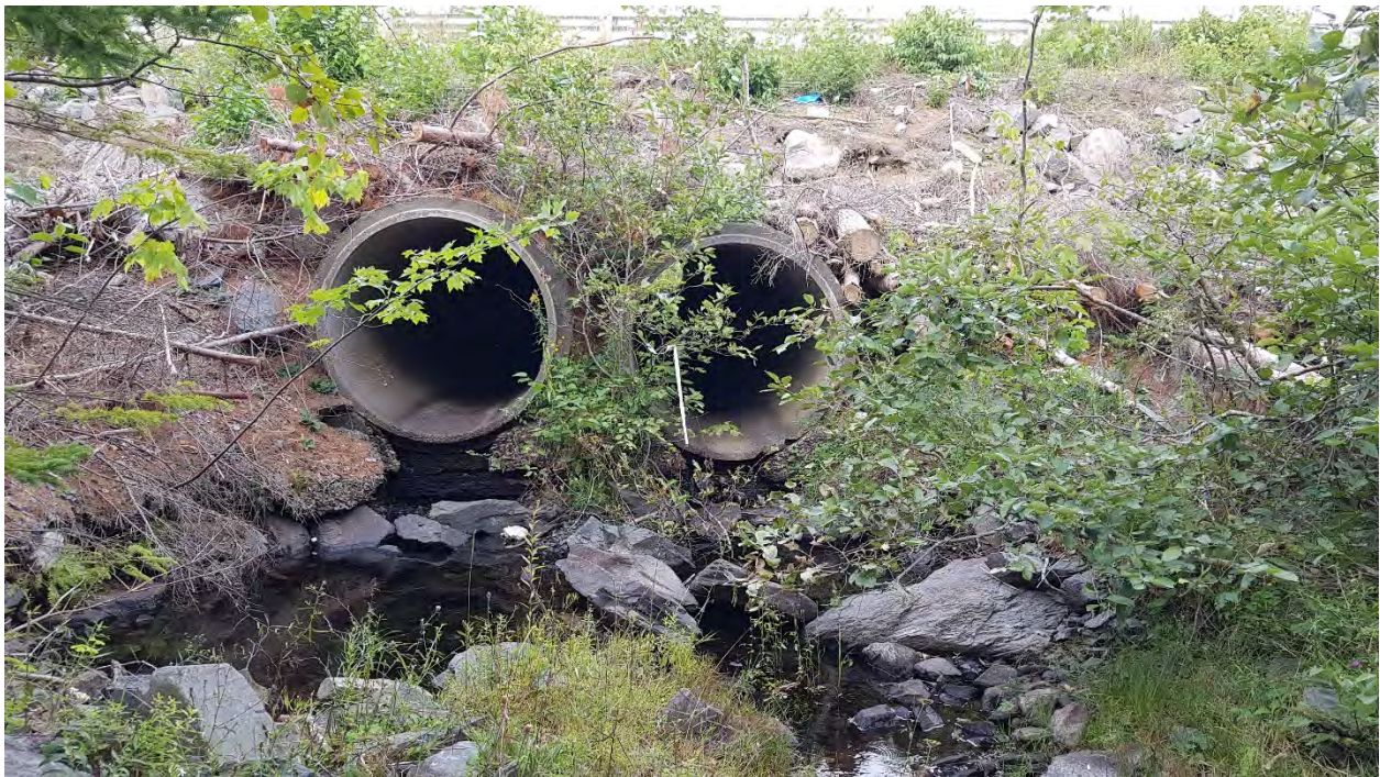
Photo 8. Area 4B – Culvert 3 has signs of seasonal high-volume flows but in July there was no flow in the culverts, although a strong current emanated from the base of the embankment.
